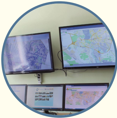
Dispatcher center (server with mnemonic) + Monitoring and control system software
