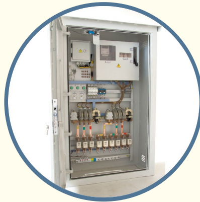
Cabinet "I-710" at the system start-up post with inbuilt lights managing terminal
