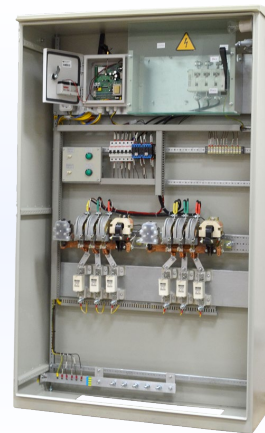
Lighting control cabinets I-710
