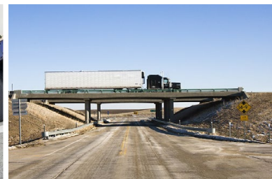
Protection of bridges
