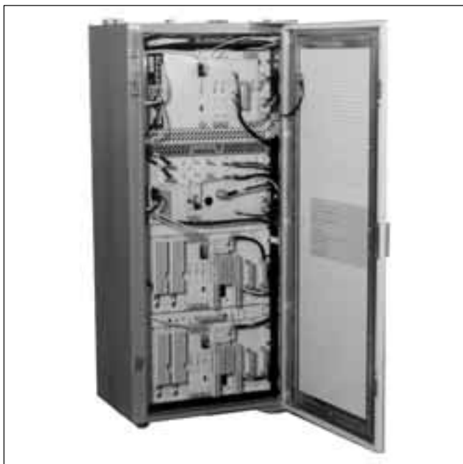
Base station of cellular network
