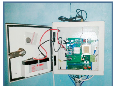
Terminal "SEA EDCS" which transmits information to the dispatcher's console via the GSM cellular network
